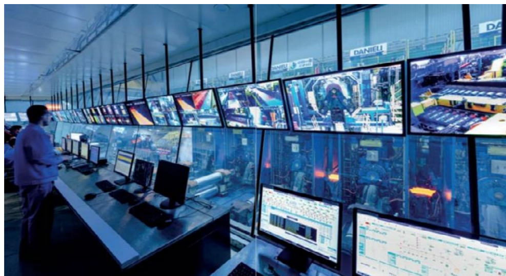
Figure 4: DUE ® control pulpit at Shougang Jingtang (P.R.China)
