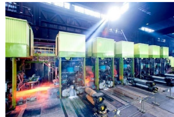
Figure 1: HSM - finishing mill section
