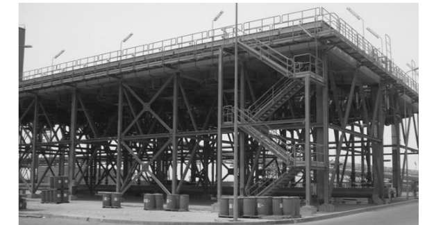
Figure 2. (Air cooled water coolers) Dry coolers
