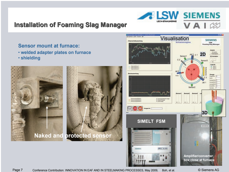
Figure 2: Example of the sensor installation at the furnace, the electric system and the visualization of the foamy slag distribution
