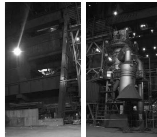
Figure 2: PEM installation at ArcelorMittal Gent
