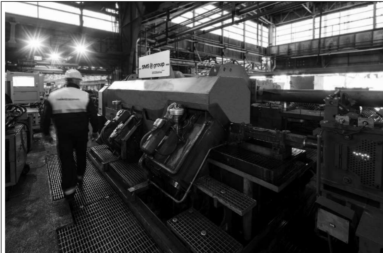
Figure 4: The MEERdrive ® PLUS in operation at Caleotto works - Italy
